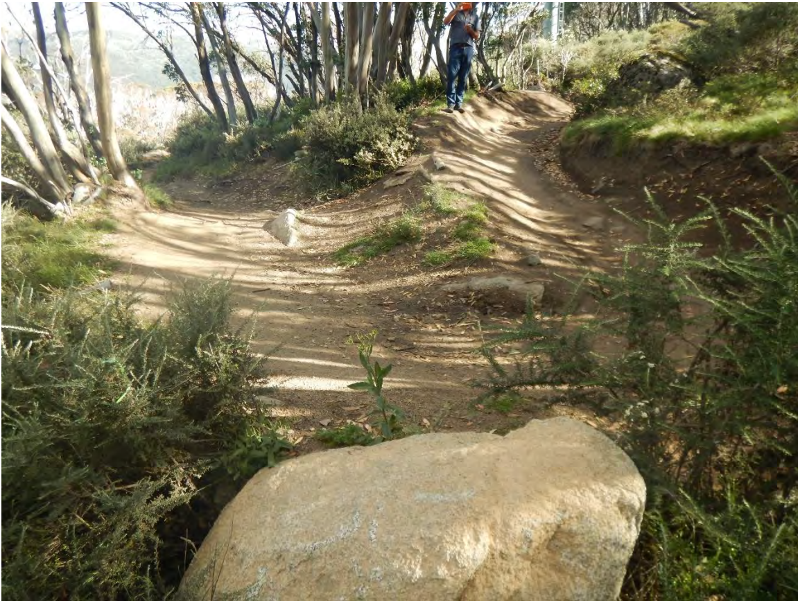
Figure 1: Section 1 – Existing corner which is too tight and technical and is to be re-aligned and rehabilitated
