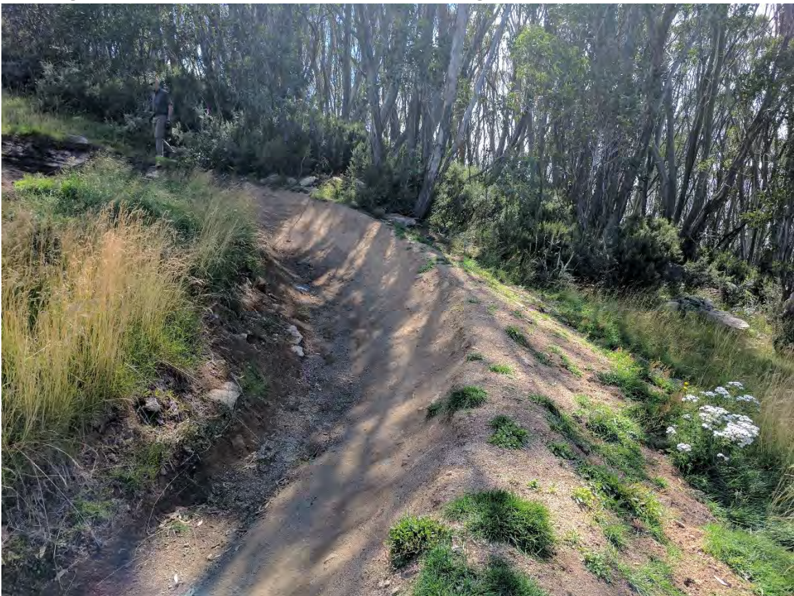
Figure 8: Section 4 – Relocation of the corner will allow for this berm to be located off the ski slope
