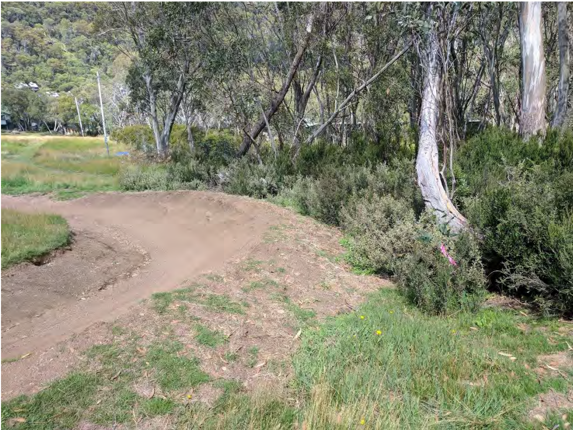
Figure 12: Section 7- Relocate corner and berm off the ski slope into the vegetation on the side of the ski run
