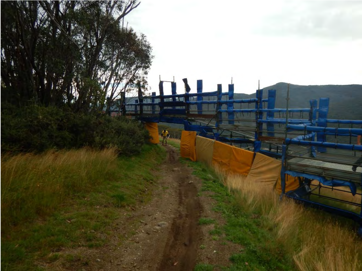
Figure 5: Section 3 - Existing temporary scaffold overpass to be replaced with a permanent structure within the tree island adjacent
